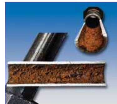
This actual cutaway of black iron air piping shows typical rust and contaminant build-up after just a few years of operation. Inside diameter may be reduced 40% over its lifetime.
